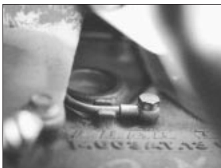
9F.19 Turbocharging oil feed pipe
